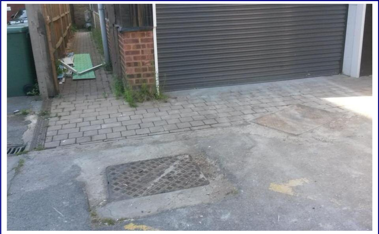
Photo 3: Surface water drain and manhole covers noted to the front of the onsite building.
