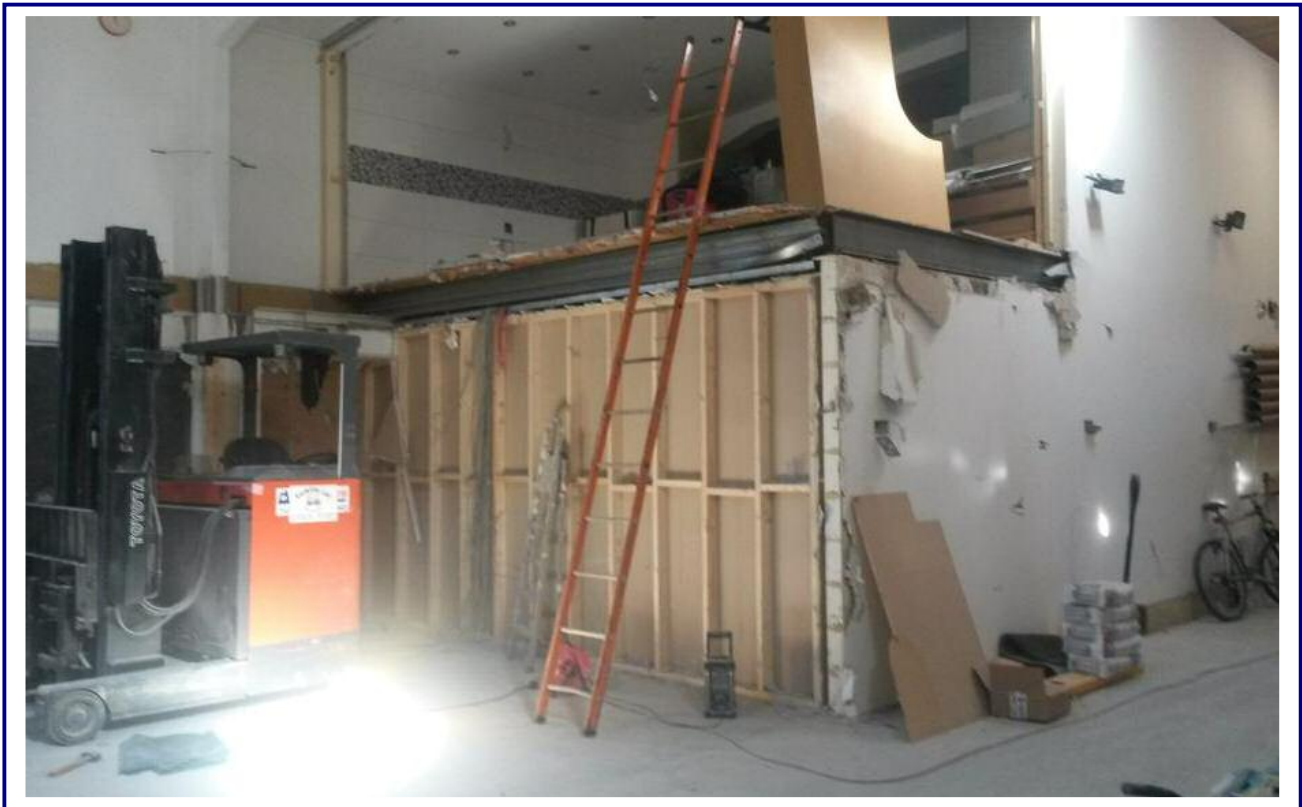
Photo 1: Warehouse area with forklift truck and ladder to former first floor show rooms.
