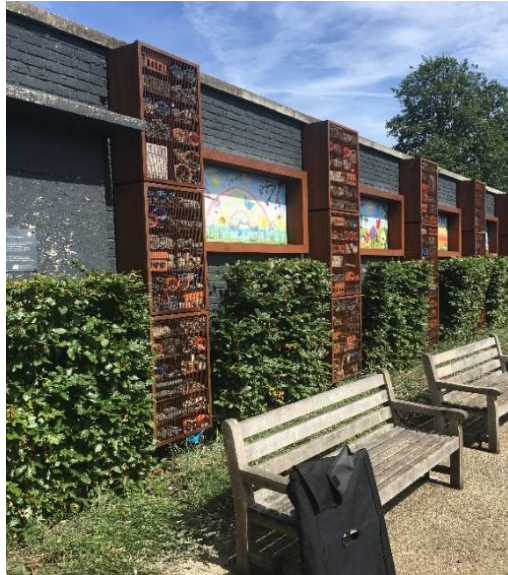
Photograph 1 Hole in brickwork on north-western elevation of Building 3
