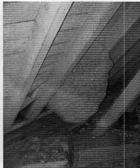
Fig. 2 Large wasp nest in roof void
