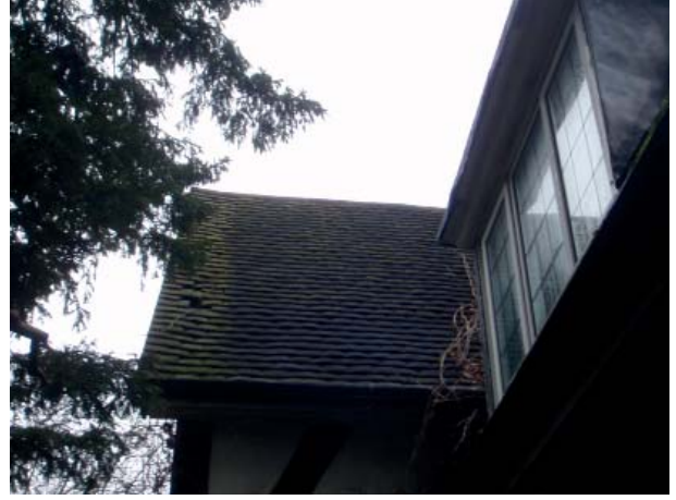
Plate 2. Section of roof with slipped/missing clay tiles.
