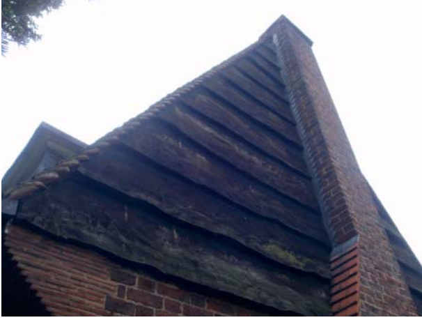
Plate 1. Weatherboarding with gaps on south-east gable end.
