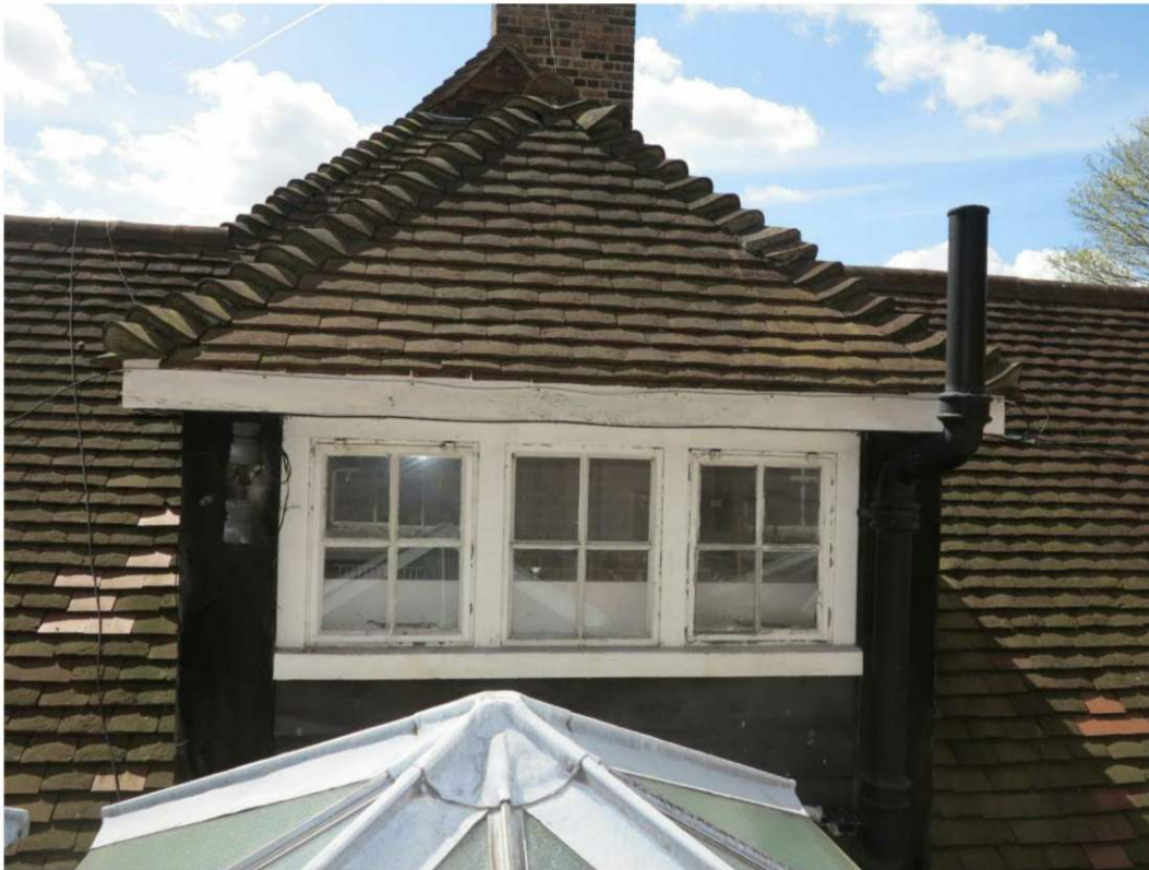
Plate 11. Hipped dormer on northern elevation of the original pavilion, as viewed from the 1960s' extension
