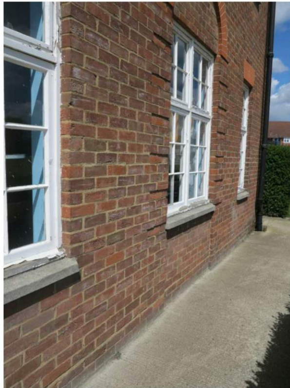
Plate 9. Roman arch to central bay of the eastern elevation of the 1960s' extension
