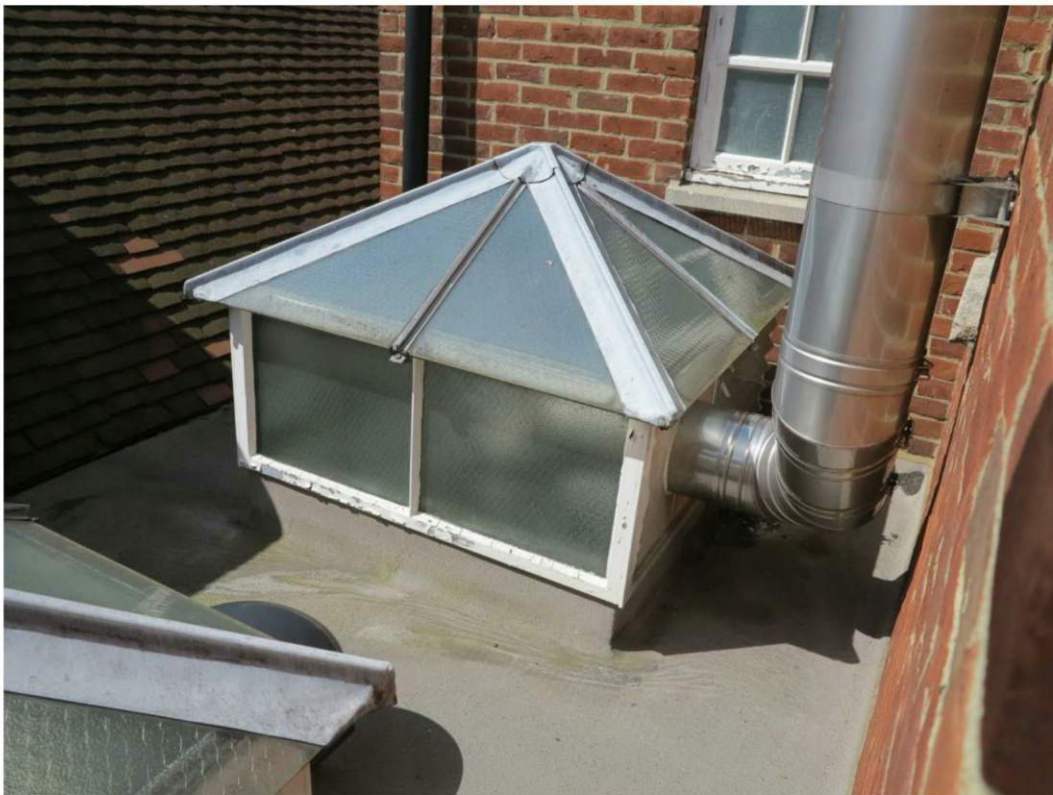
Plate 10. Flat-roofed infill between the main portion of the 1960s' extension and the original pavilion
