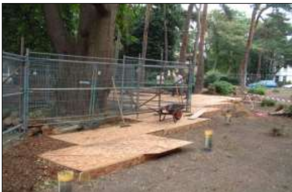
New structure image 7: Once the piles have been installed (yellow tops), the ground protection to support the piling rig is removed ready to fix the void-former onto the bare soil, in advance of pouring the building slab.
