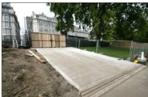
New surfacing image 8: This temporary access for heavy construction traffic on the outer edge of a RPA is a concrete slab cast above ground level and will be removed when the project is completed.
