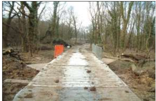
Ground protection image 6: Custom designed sectional tracks can be joined to support very heavy traffic use through sensitive areas.
