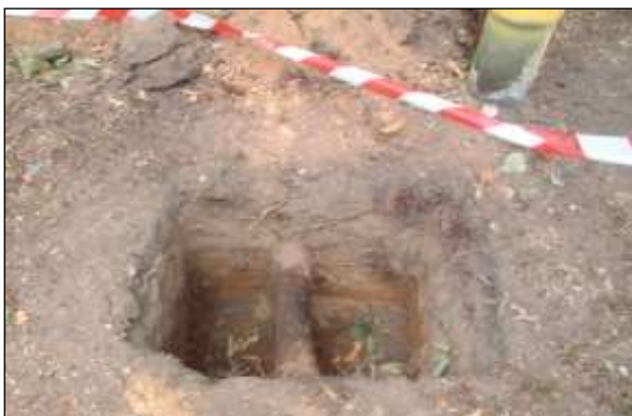
New structure image 5: Where piles are proposed close to trunks, it is essential to excavate 50–75cm deep to see if there are any significant roots in the way, with provision to move the pile location if roots are found (note the pile was finally installed to avoid this root).
