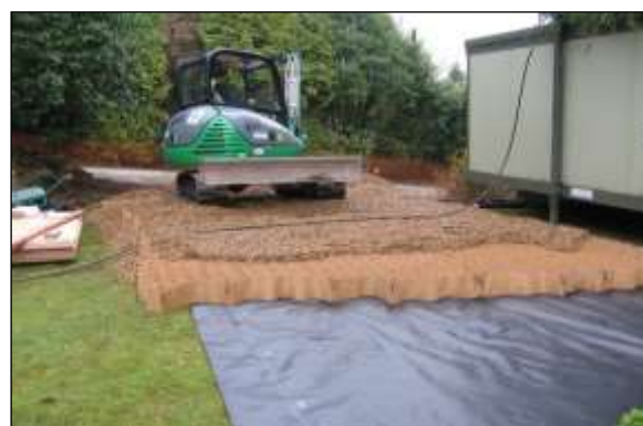
New surfacing image 3: The stone-filled cells spread the load of traffic and the geotextile membrane on the ground prevents migration of the stone into the soil profile.
