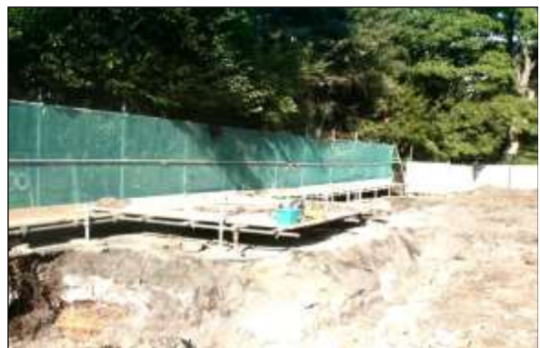
Ground protection image 4: A scaffold framework attached to the main scaffold fencing can be used to support either scaffold planks or plywood to create an elevated platform with a gap beneath.
