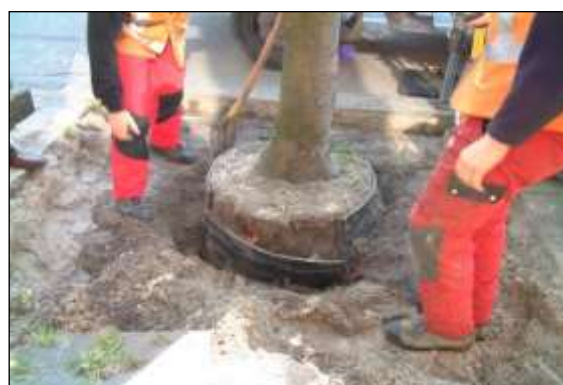
Soil cell image 4: This excavated tree shows the root deflectors that were installed when it was planted seven years previously. The product has deflected roots downwards and prevented damage to the adjacent surfacing. Note that this is a permeable sandy soil and the roots were able to grow beneath the bottom of the deflectors.
