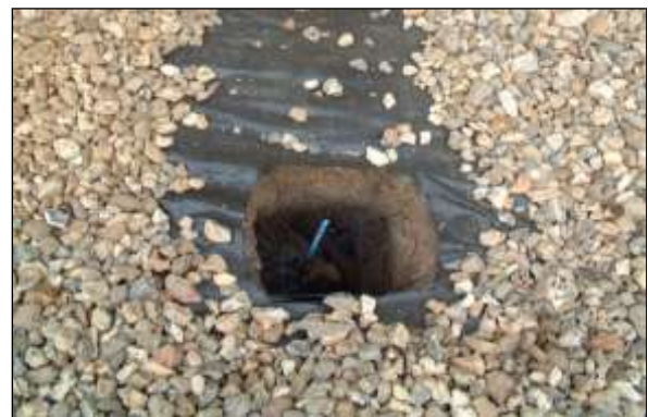
New structure image 6: Ground protection must be used to spread the load of the piling rig once excavation has confirmed that no substantial roots are in the preferred pile location.
