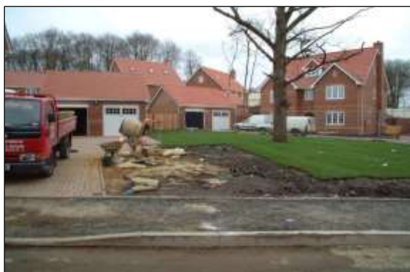
Landscaping image 1: The RPA of this tree was not effectively protected during construction and excessive compaction of the soil meant it died soon after this turf covered up the damage.
