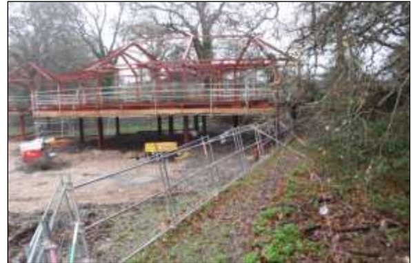
New structure image 4: It is possible to support very large structures on piles within sensitive RPAs without any significant adverse impact on tree roots.
