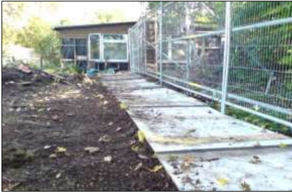
Ground protection image 1: Heavy-duty plywood set onto a compressible woodchip layer and pinned into position is suitable to spread the loading from pedestrian access.
