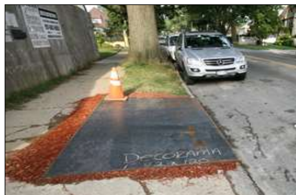
Ground protection image 8: Steel plates can be an effective way of temporarily reinforcing weak surfacing over a construction access during the development activity.
