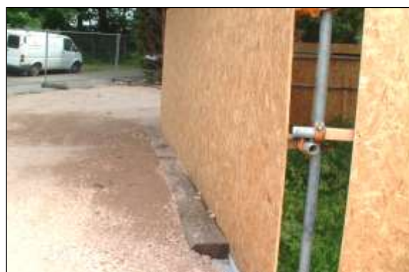
New surfacing image 5: Although this is only a temporary surface, railway sleepers pinned into the ground can be used to retain the edges of new surfacing.
