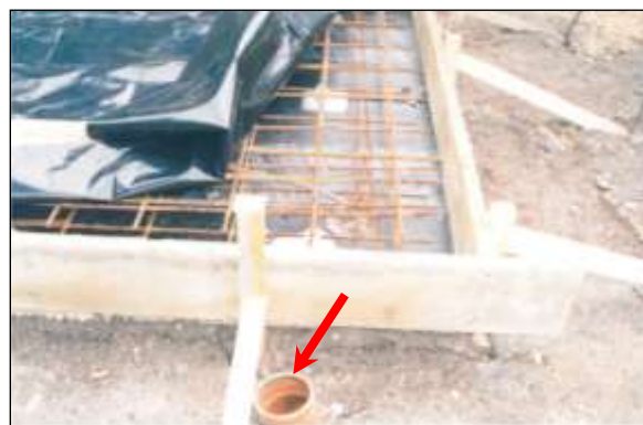
New structure image 10: This reinforced base slab for a double garage has drainage provision (red arrow) beneath the structure to redirect roof runoff to supply roots with water.
