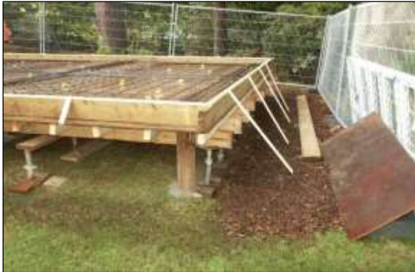
New structure image 3: Small diameter piles (less than 150mm) are an effective means of supporting structures in RPAs with minimal disturbance.
