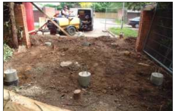
New structure image 8: Piles can also be used to support bridges across sensitive RPAs, but the temporary ground protection has to be removed before the main structure is either imported in or cast on site.
