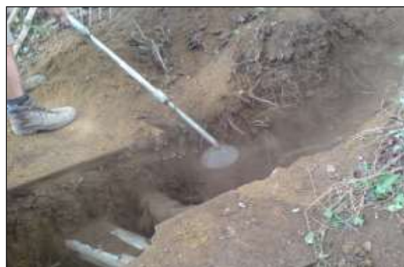
Excavation image 2: Air spades are very effective at exposing roots and services with minimal damage.
