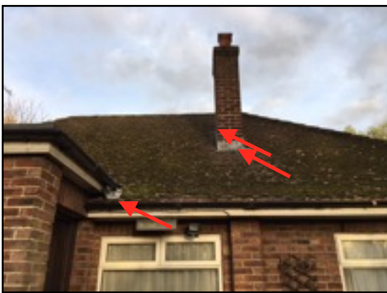
Image 8: West facing elevation of the house. Arrows point to missing tile and gaps under the lead flashing.
