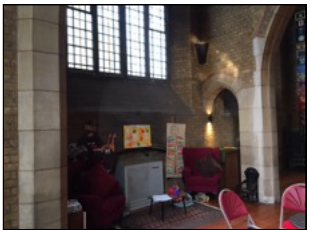
Figure 15: The internal wall where the church will be linked to a new corridor linking it to the hall. No evidence of bats was found in this area.
