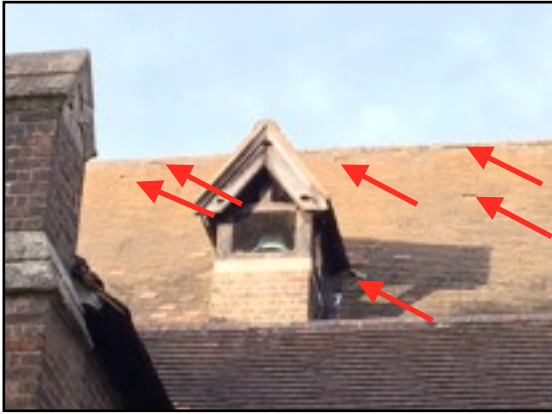
Image 6: Church roof, east elevation. Arrows point to missing tiles and gaps.
