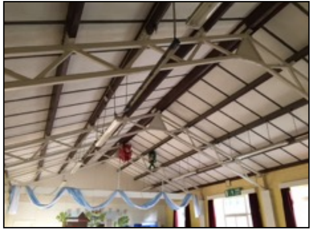
Figure 11: Internal roof of the hall, other sections of the building had no voids only plastered ceilings.
