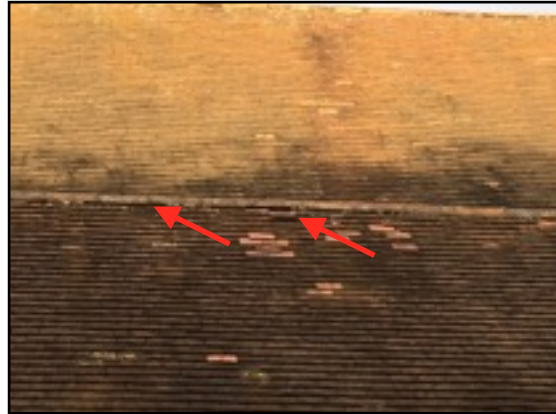
Image 7: Church roof, east elevation. Arrows point to missing tiles and gaps.
