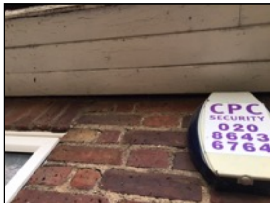
Image 9: No gaps visible under the soffit boards of the bungalow.
