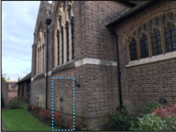
Figure 16: The external section of the wall whereby the corridor will enter the church.
