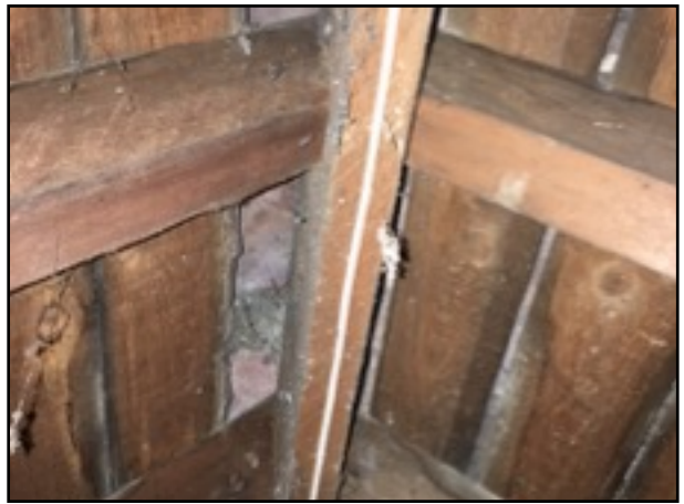
Figure 13: Timber behind the tiles with some cobwebs.
