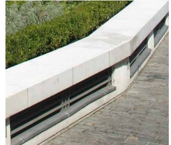
Integrated basement ventilation
