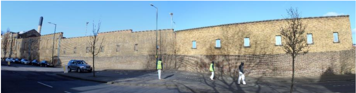
Figure 43: External elevation of south boundary wall with section 1 (left end) and section 2 (right end)
