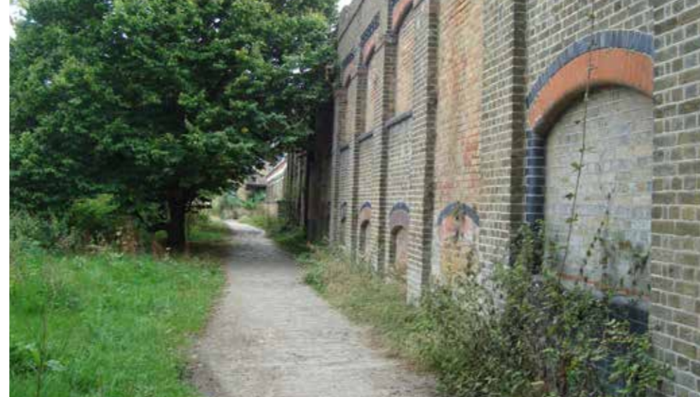
Photograph 4 - View of towpath and existing River Wall forming the north east boundary of the Stag Brewery component of the Site.
