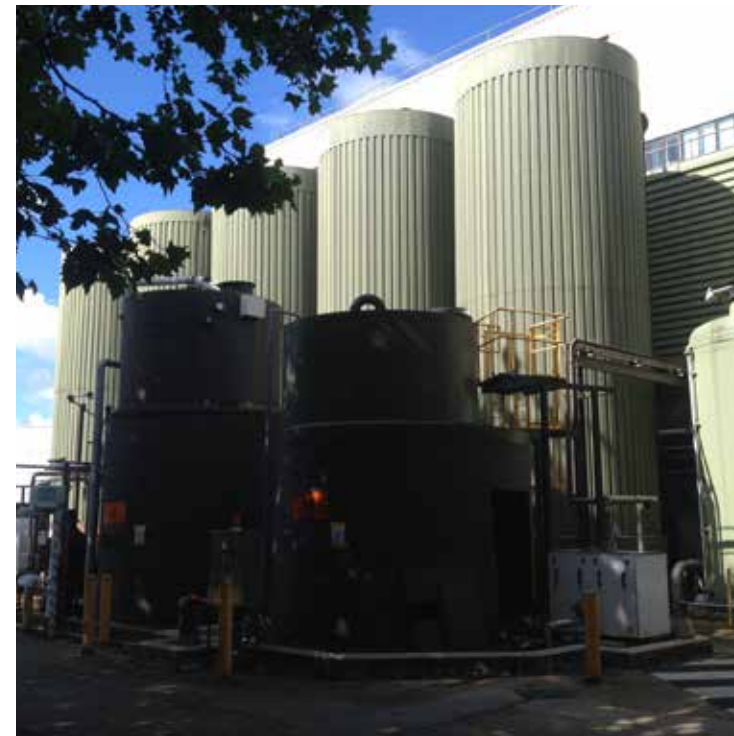
Hydrochloric acid, caustic soda, salt and water tanks adjacent to Brewhouse
