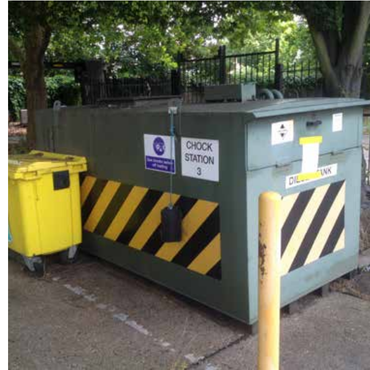
Diesel tank in Packaging Warehouse yard
