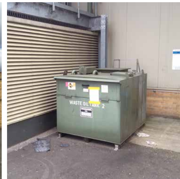
Waste oil tank at Packaging Warehouse
