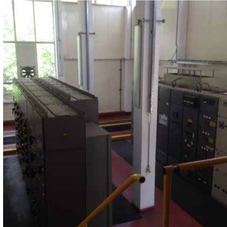
Electrical infrastructure within Energy Centre
