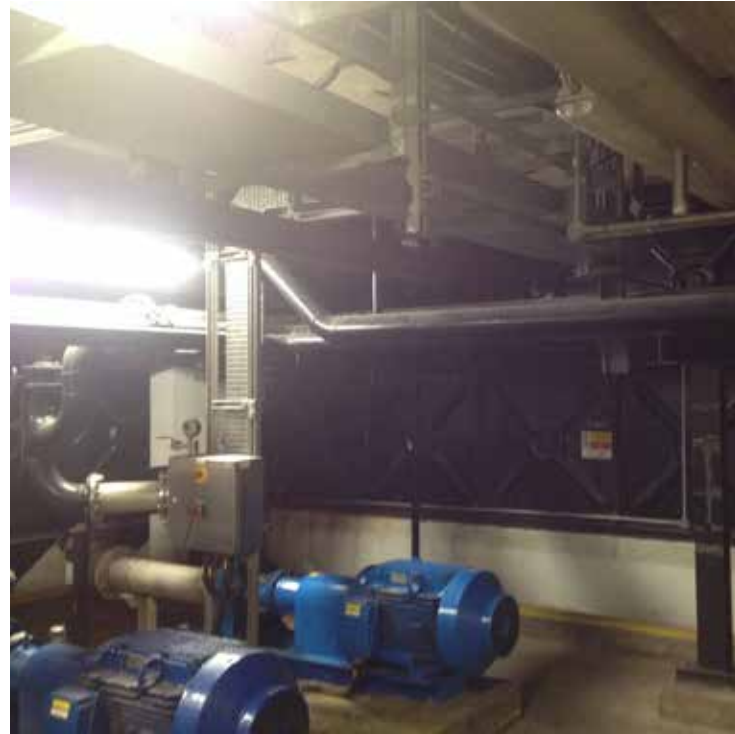
Water tanks and pumps in Production Office basement
