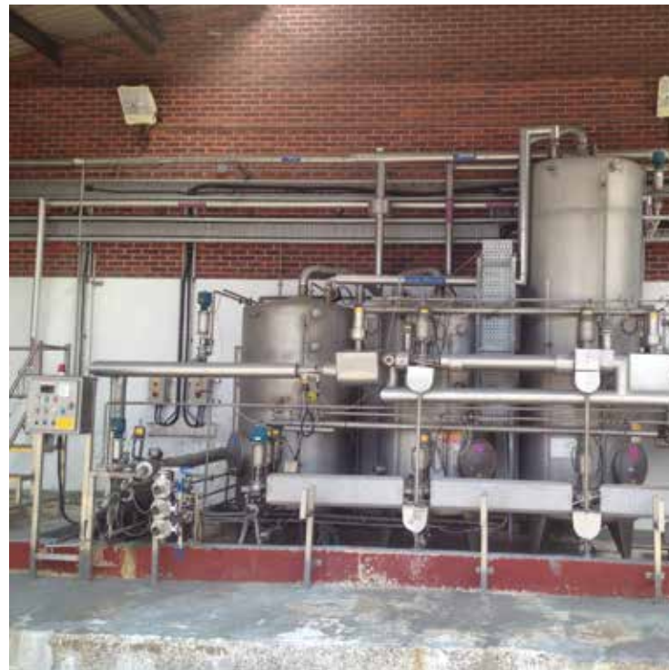
HCl, caustic soda and LCT tanks at maintenance building
