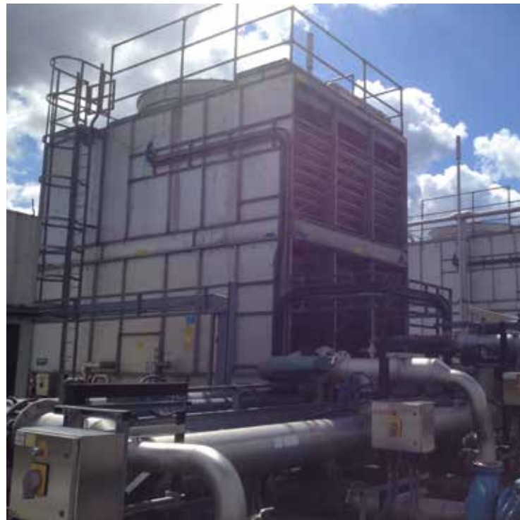
Air conditioners at Energy Centre roof
