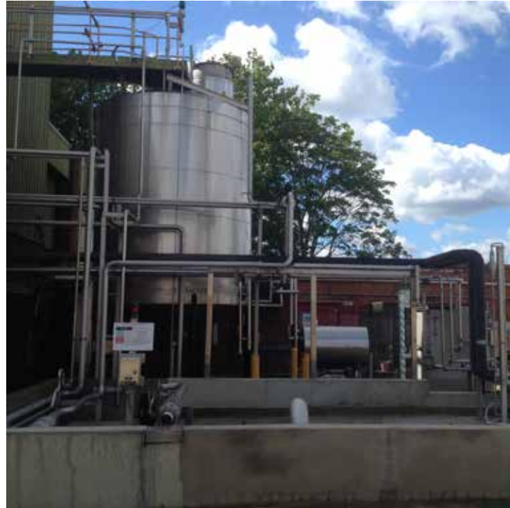
Waste yeast tank and chemical stores
