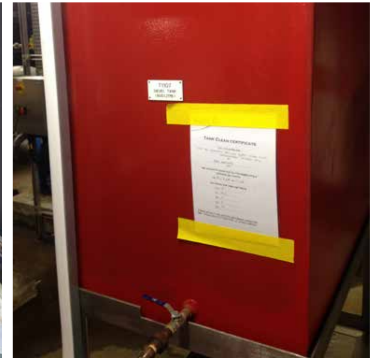
Decommissioned diesel tank in Production Office basement
