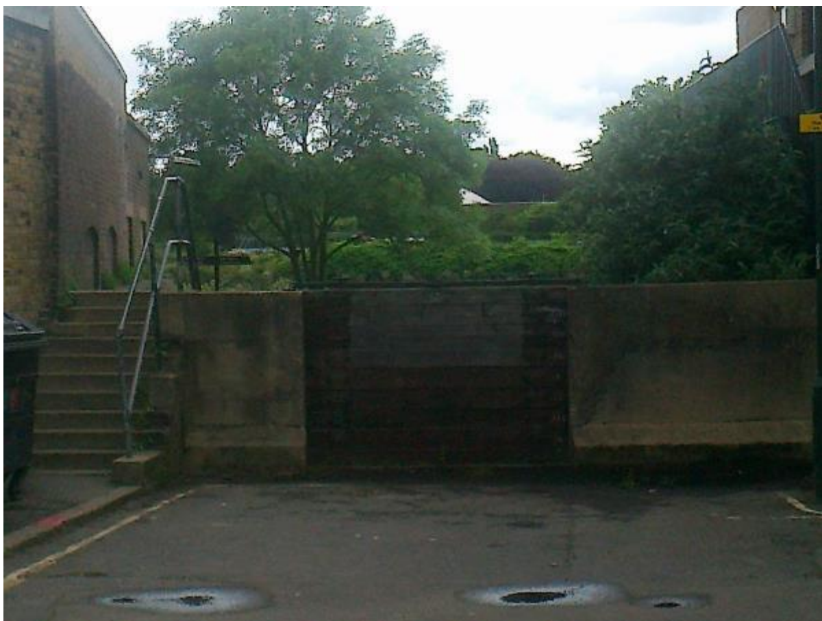
Figure D-4 Stop-Logs at Bull's Alley (towards river)
