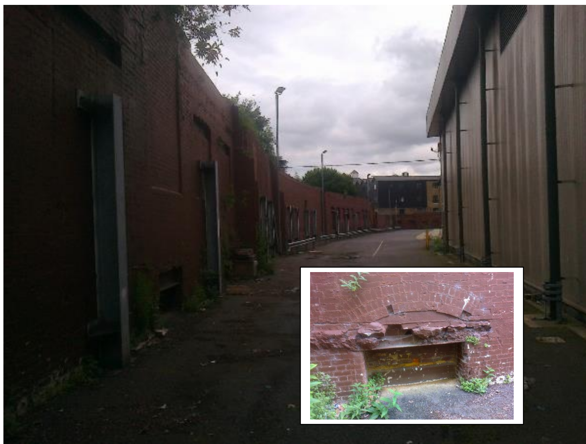
Figure D-2 Existing tidal defences (inset shows bricked up window)
