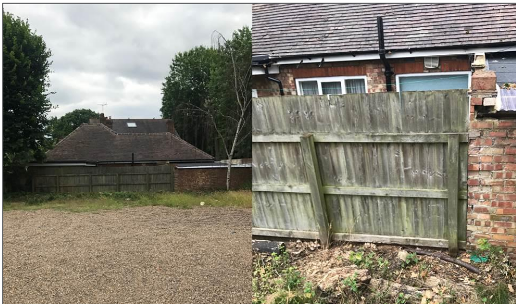
Figure 7: Site survey photo of the north façade of the affected neighbouring building
