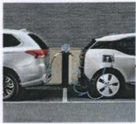
Typical 2 car charging pole
