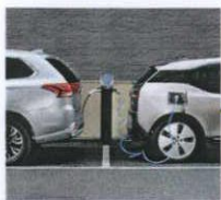
Typical 2 car charging pole
