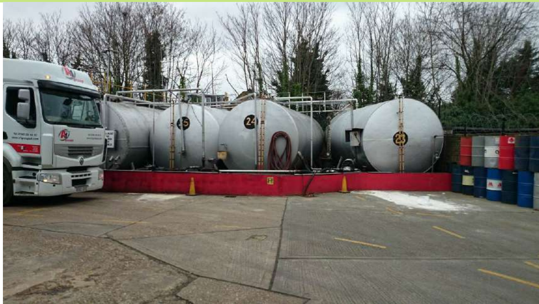
Plate 15 – Northern end of tank farm
