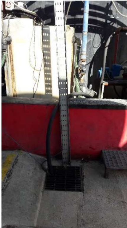
Plate 9: Sump pump forming part of the engineered drainage system
