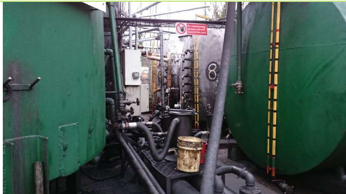
Plate 17 – Looking into tank farm, black staining within bunded area.
