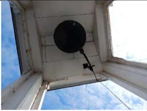
A view of the bell tower situated above the loft space hatch in the kitchen area of the southernmost apartment. A hole can be seen in the underside of the bell mechanism housing, revealing a possible void within.
