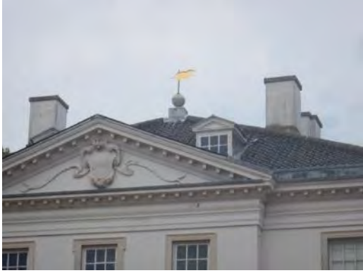
Close up view of dormers showing possible gaps
