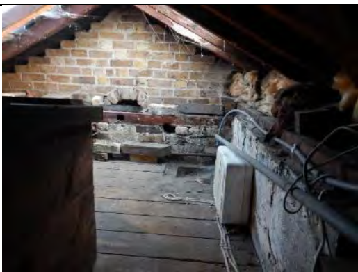
A view of the small loft space to the east of the main loft space described above, with the brick wall to the rear of the photo housing the clock face.
