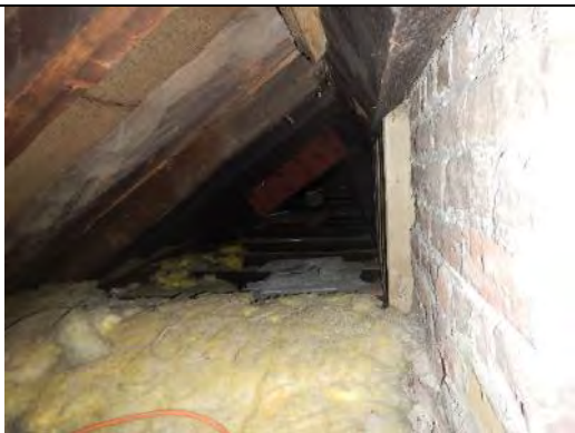
View of the eave roof spaces which extend the length of the southern elevation and link with the West and East Garret at either end.
