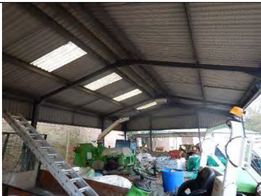
A view from inside the main plant storage building, showing the open sides to the building, corrugated metal sheet roofing, steel frame structure and the netting on underside of roofing to prevent access to birds.
