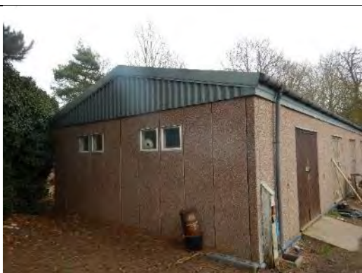
The Western facade of the maintenance building showing the concrete walled and corrugated metal roof structure of the building.
