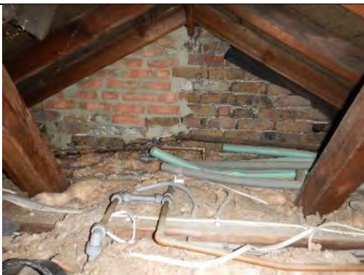
The brick firewall positioned to the north of the loft space with a missing brick shown to the right of the photo, revealing the loft space beyond.
