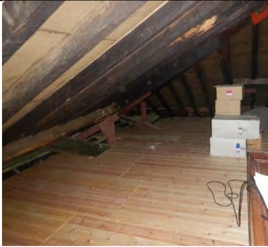
Context view of one of the two boarded roof spaces, i.e. the East Garret and West Garret.
