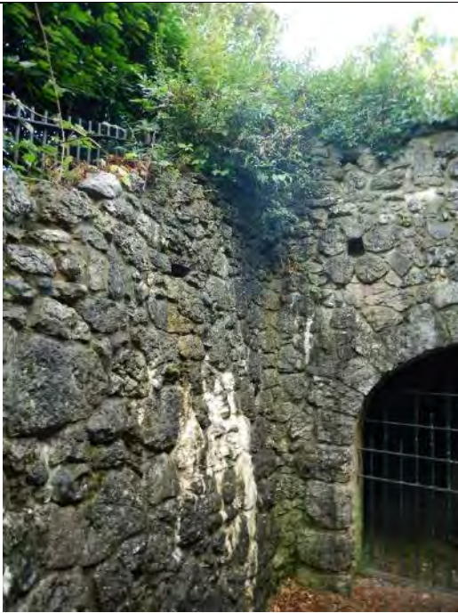
View of the stone-work at the entrance to the grotto which possesses numerous crevices
