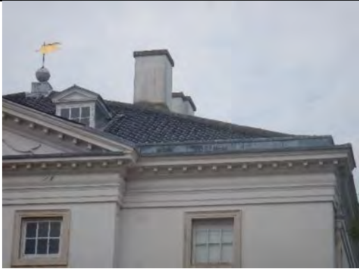
Close up view of possible slight gap between mortar and hip tiles / upper most roof tile
