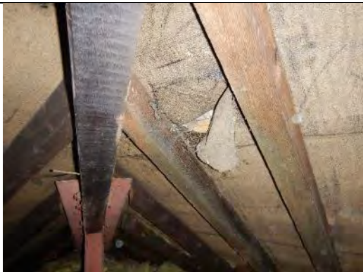
Close up view of a section of torn bitumen roofing felt liner towards the southern end of the East Garret, through which the roof tiles and daylight were visible.
