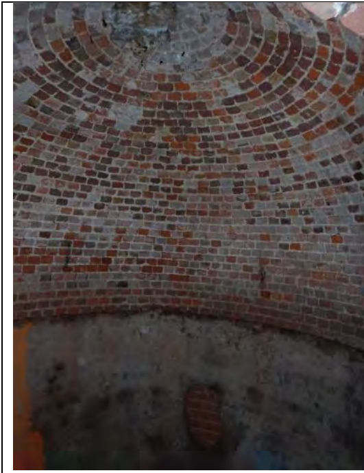
View of the domed ceiling of the sunken ice house section, again with intact mortar
