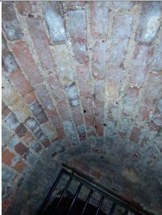
Close up view of the brickwork ceiling of the ice house passageway showing intact mortar and several spiders
