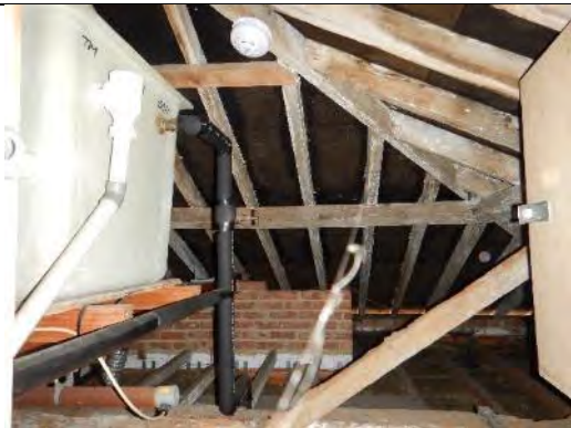
A view of the water tank above the men's toilets in the rear extension of the coach house.
