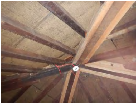
Close up view of timber joints at apex of the hipped roof.
