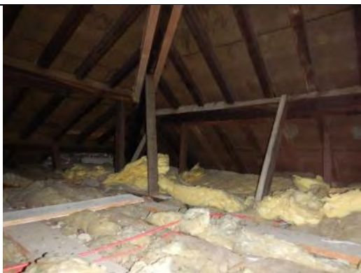
View of the unboarded loft space showing how trusses are limited to the peripheries, providing an uncluttered flying space
