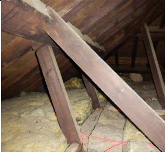
View of exposed timber and bitumen lines roof slopes with insulation and occasional exposed joist; large wasps' nest in background
