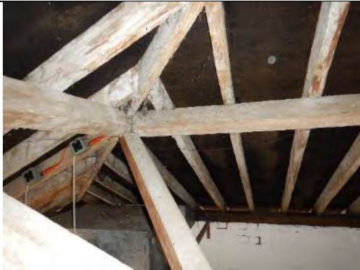
View of the northern rear extension of the coach house showing the timber framed roof with felt lining.
