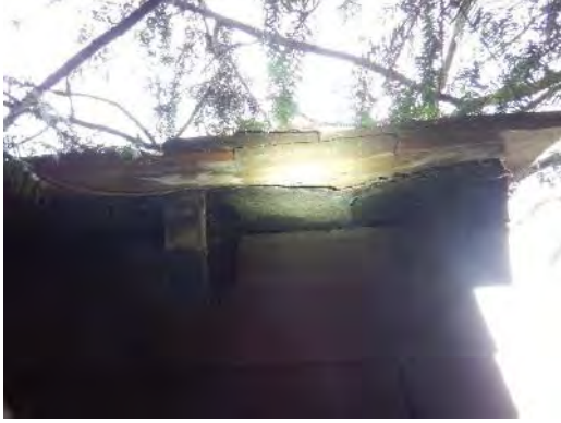
A picture showing a gap at eave level of the coach house store building.
