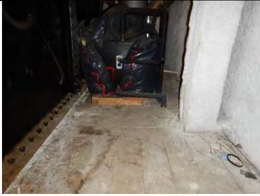
A view of the plant room loft space floor with the water tank shown to the left.
