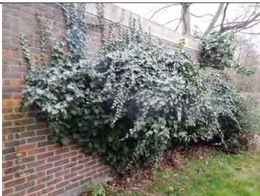
A view of parts of the ivy covering the south-west section of the main parks office building containing disused birds' nests.
