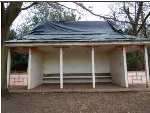
A picture showing the front of the pagoda building with the wooden frame structure and tarpaulin covered roof.
