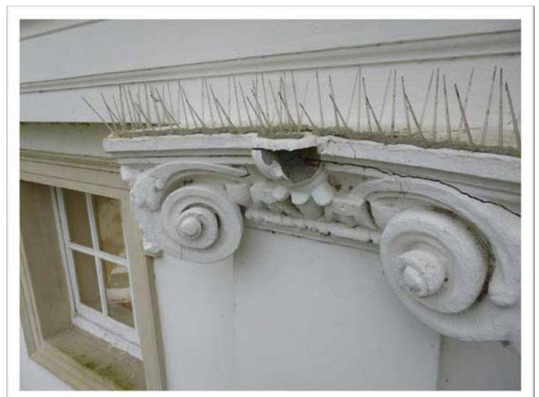
Fig. 17 Marble Hill House, decaying north pediment capital.
