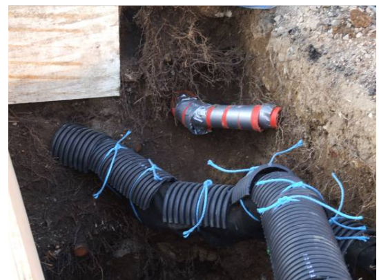
Photograph 3: Exposed roots protected from damage with wet Hessian and split plastic pipe
