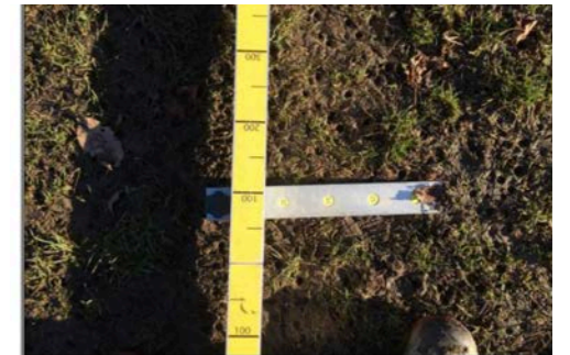
Plate 14: Undulation > 25mm depth – centre circle
