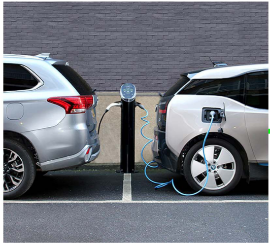
Typical 2 car charging pole
