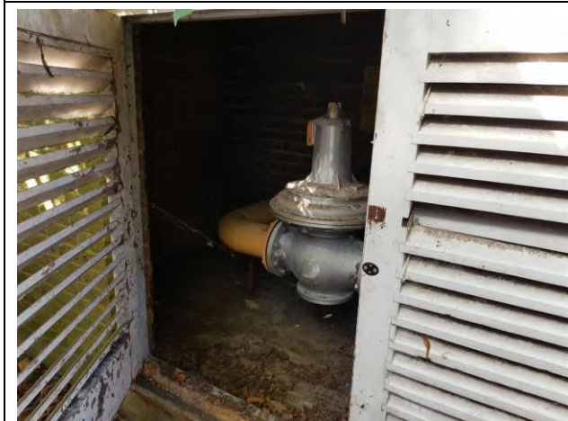
Gas service cupboard on northern boundary.
