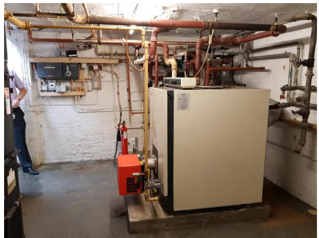
Plant room still in use under Beatrice Lodge , with former tank base.
