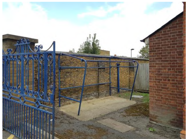
Asbestos roof has been removed from bike shed adjacent to the Porters Lodge .
