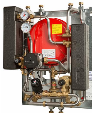
Typical HIU in each apartment:
