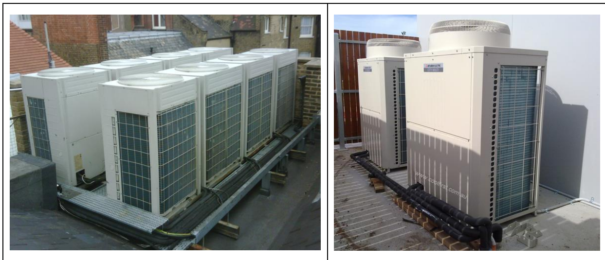
Figure 20: Typical VRF installation showing external condensing units on roof and on ground level
