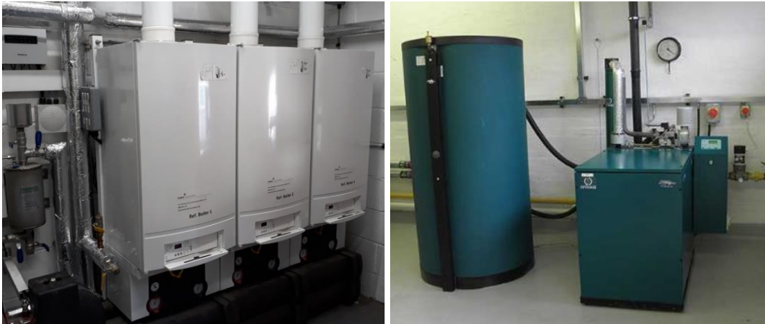
Figure 12: Illustrative communal heating plant containing LTHW boilers and micro-CHP (for residential blocks)
