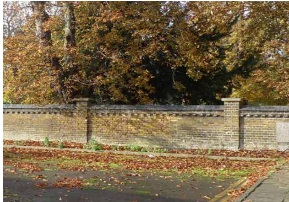
Figure 5.9 The boundary wall between the Site and the Old Mortlake Burial Ground. The wall is broken down in places and in a low to poor overall condition.
