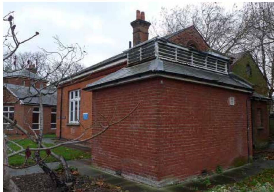
Figure 4.2 The later additions and alterations to the east elevation of the Recreation Hall (1903-4).
