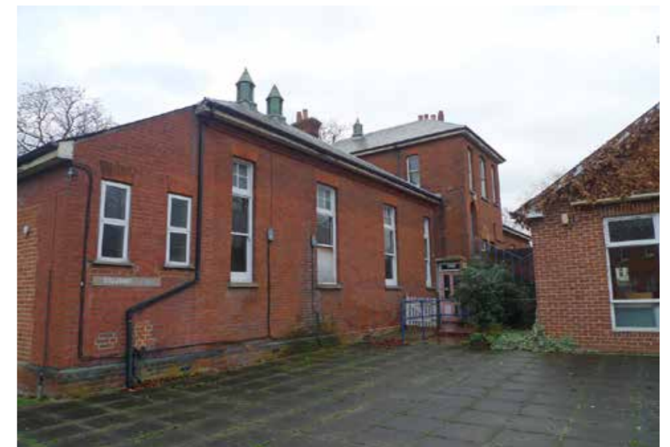
Figure 4.6 Elizabeth Lodge, 1903-4, east elevation, showing alterations to the access to the central bay to provide a new access and connection to the later building to the east.
