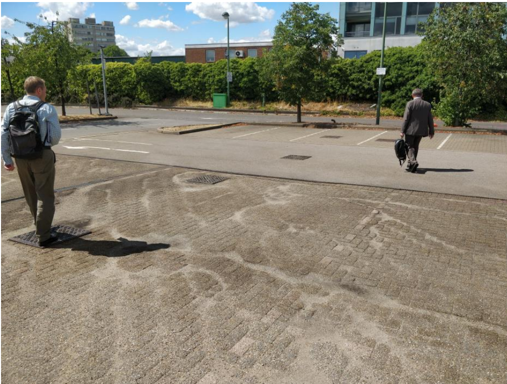
Photo 4: Area of paving and possible interceptors at assumed location of former car park
