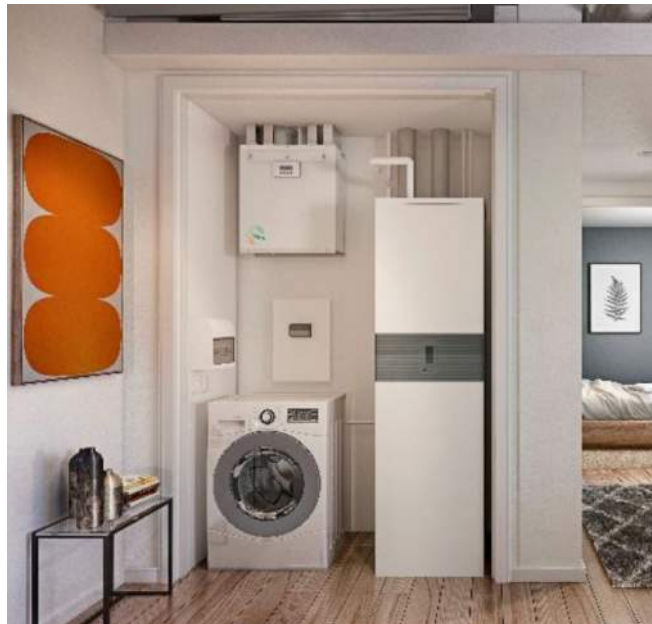
Figure 2 – A heat pump and hot water cylinder within an apartment utility cupboard
