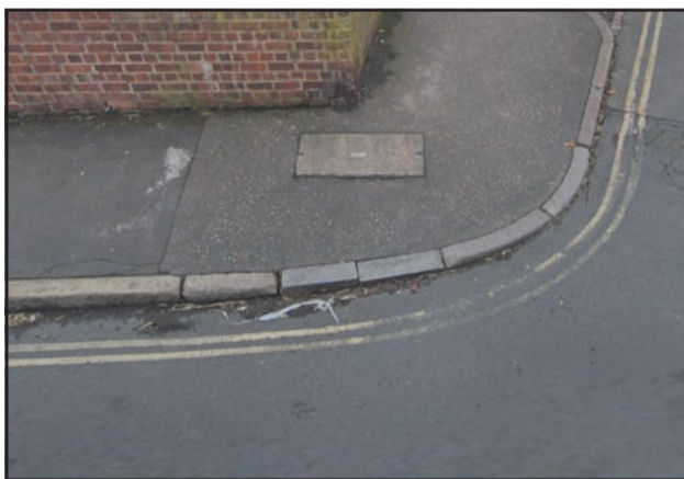
Kerb damage on corner of Edwin Road and Marsh Farm Road
