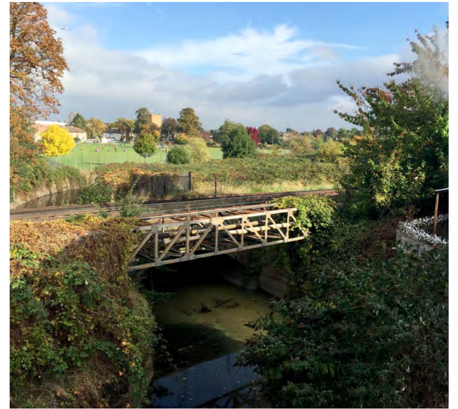
9. The railway bridge and the view of playing fields to north of site
