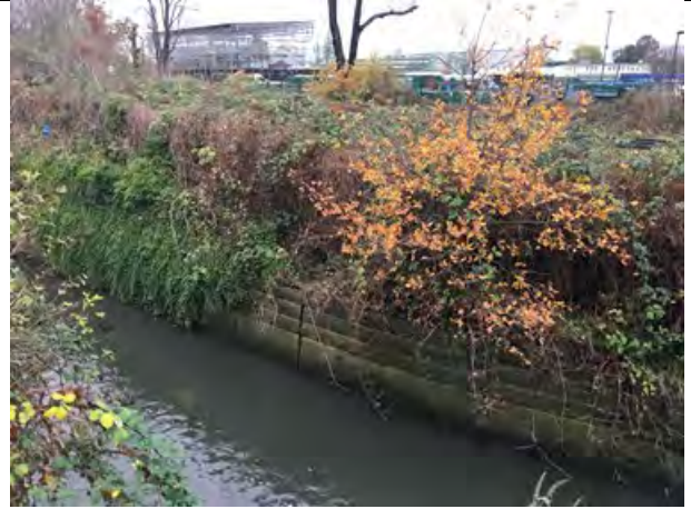
Photo 12: River Crane to the north of the site reinforced with concrete sides
