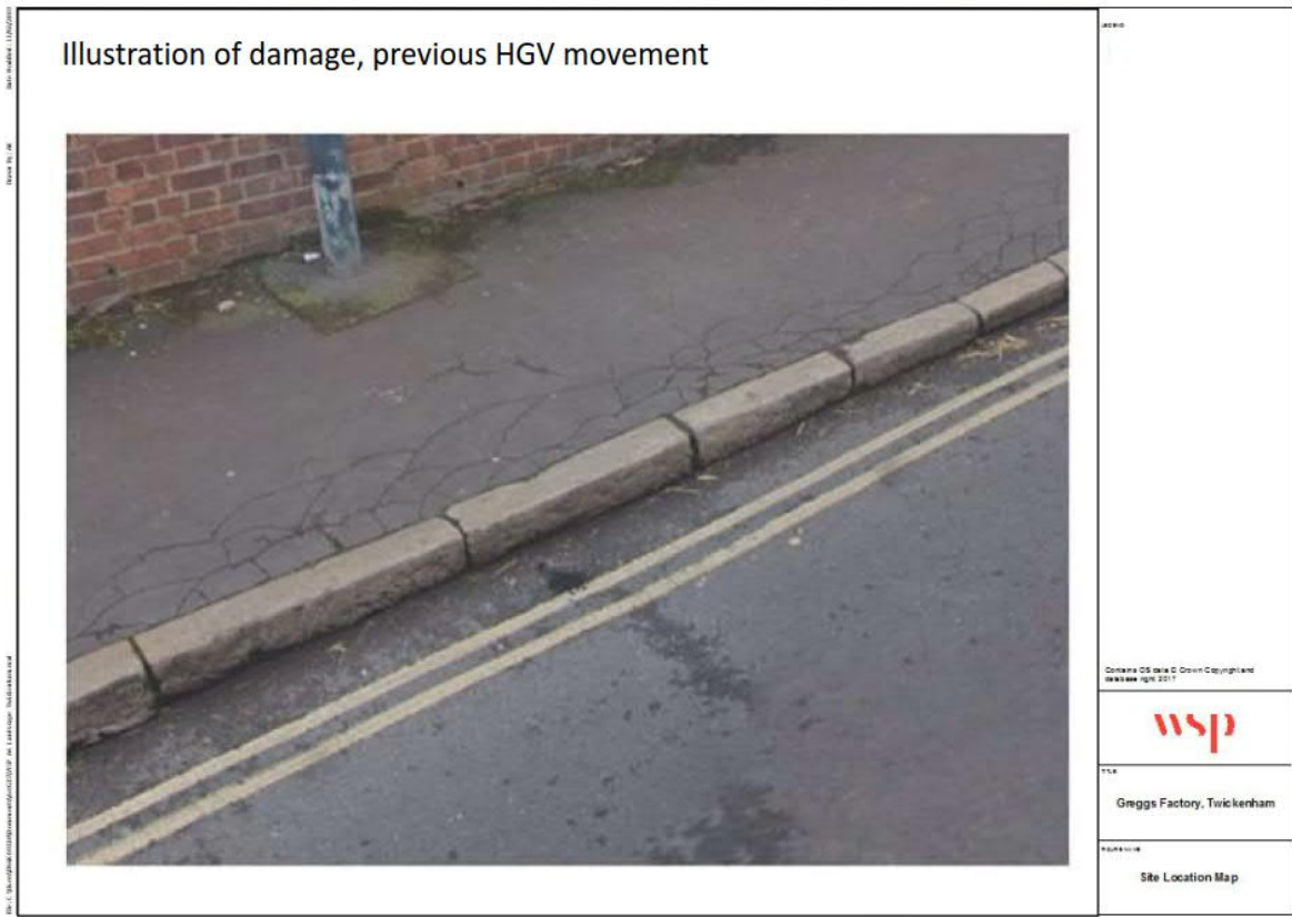
Figure 5-2 - Illustration of damage, previous HGV movement
