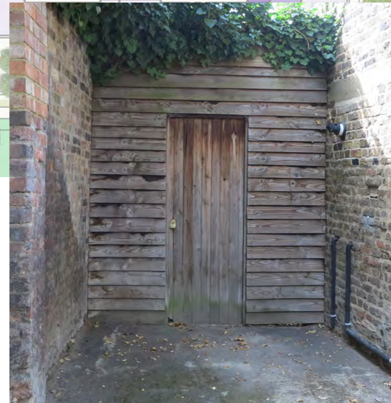
Photograph showing obstruction to shared access route
