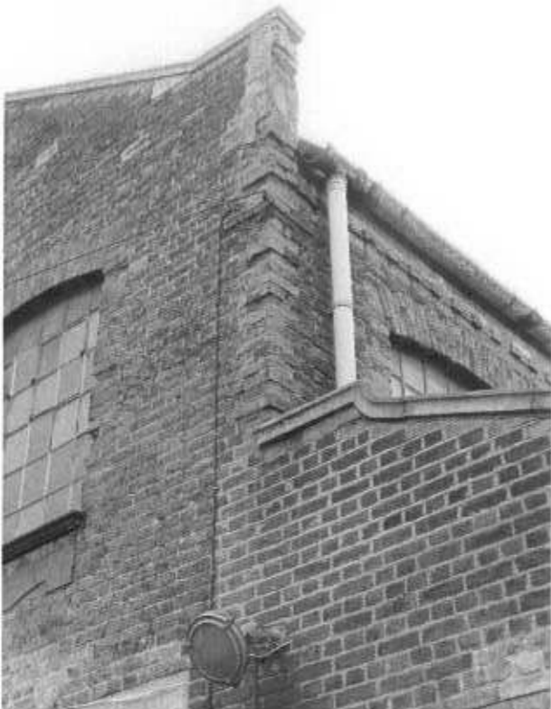
BUILDING 3 - CONDITION OF SOFT RED BRICKWORK
