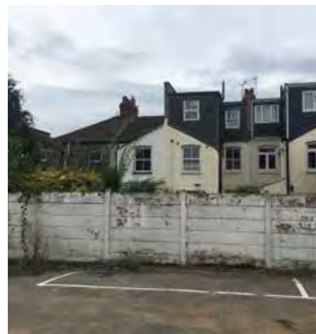
Boundary wall to be retained to the rear of Gardens of Gould Road
