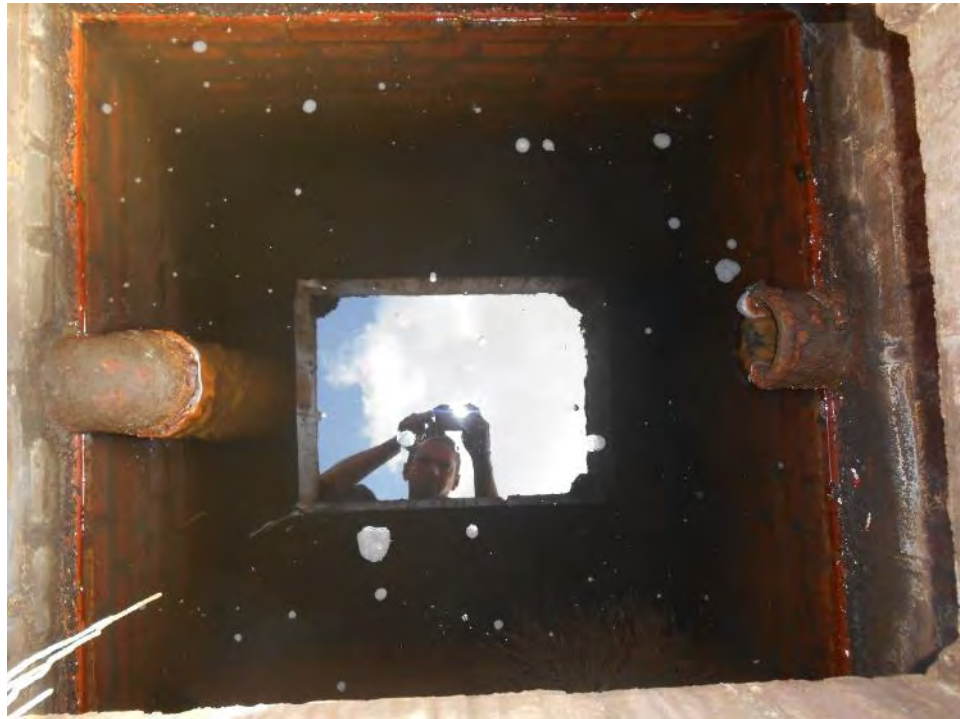
Photo 33: Conditions inside the interceptor
