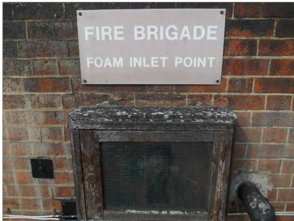
Photo 14: In case of fire facilities
