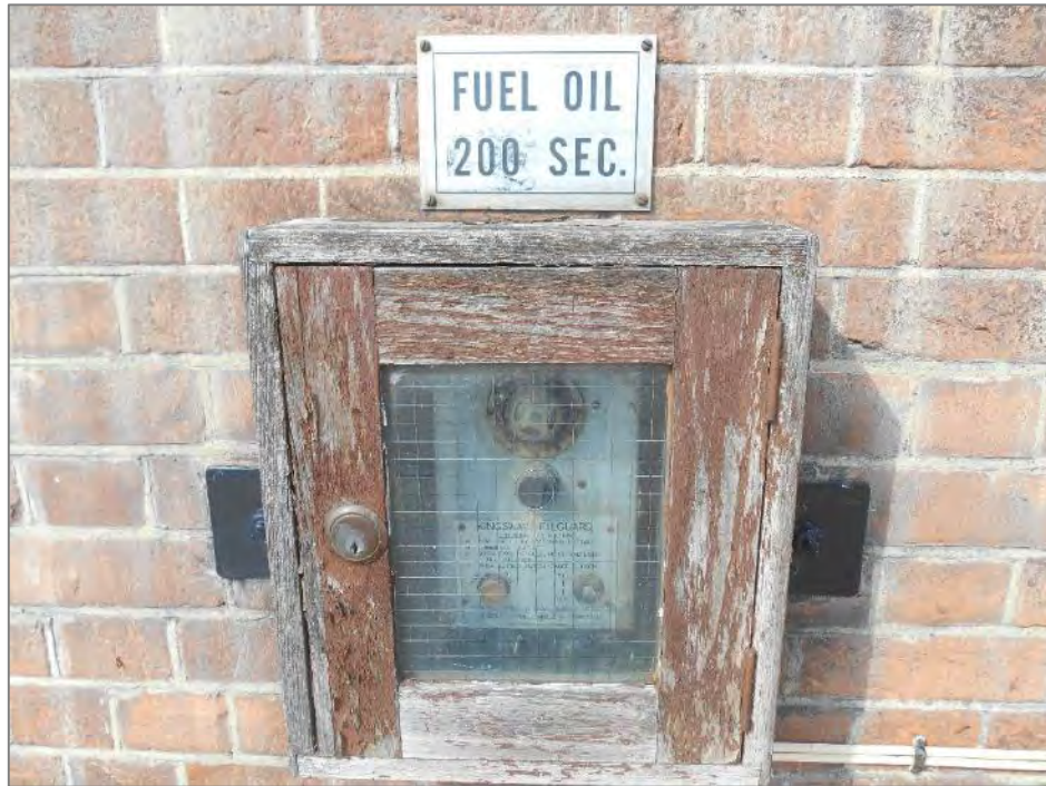
Photo 13: Fuel oil dispenser
