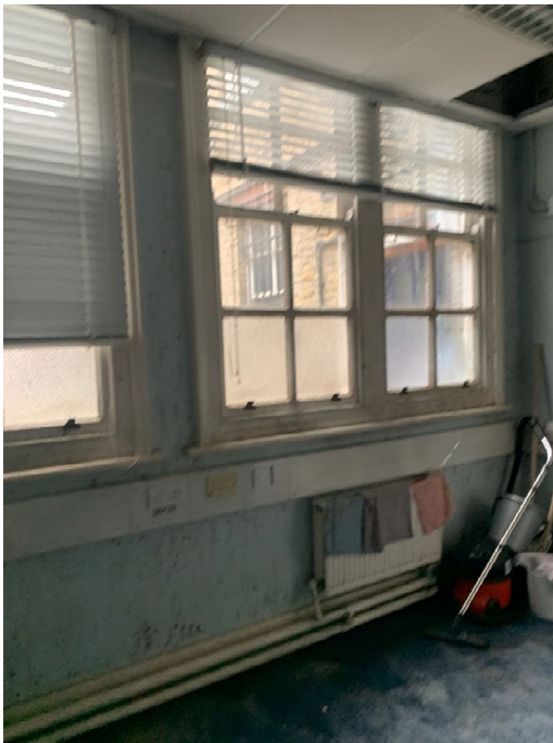
10. Rear wall of single storey extension indicating damp
