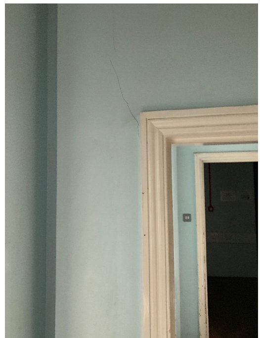
11. Typical example of cracking to plaster
