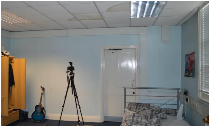
A plain original door within a much-altered room on the ground floor.
