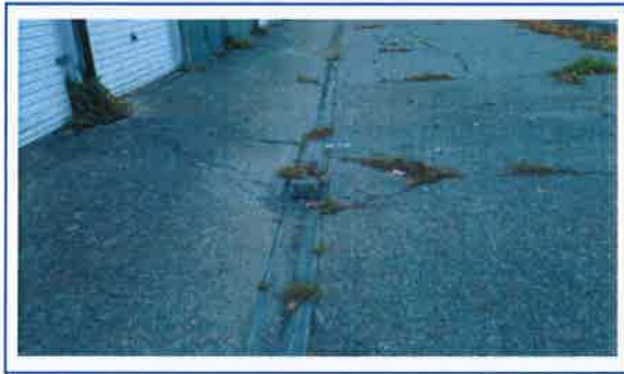
Condition of hardstanding
