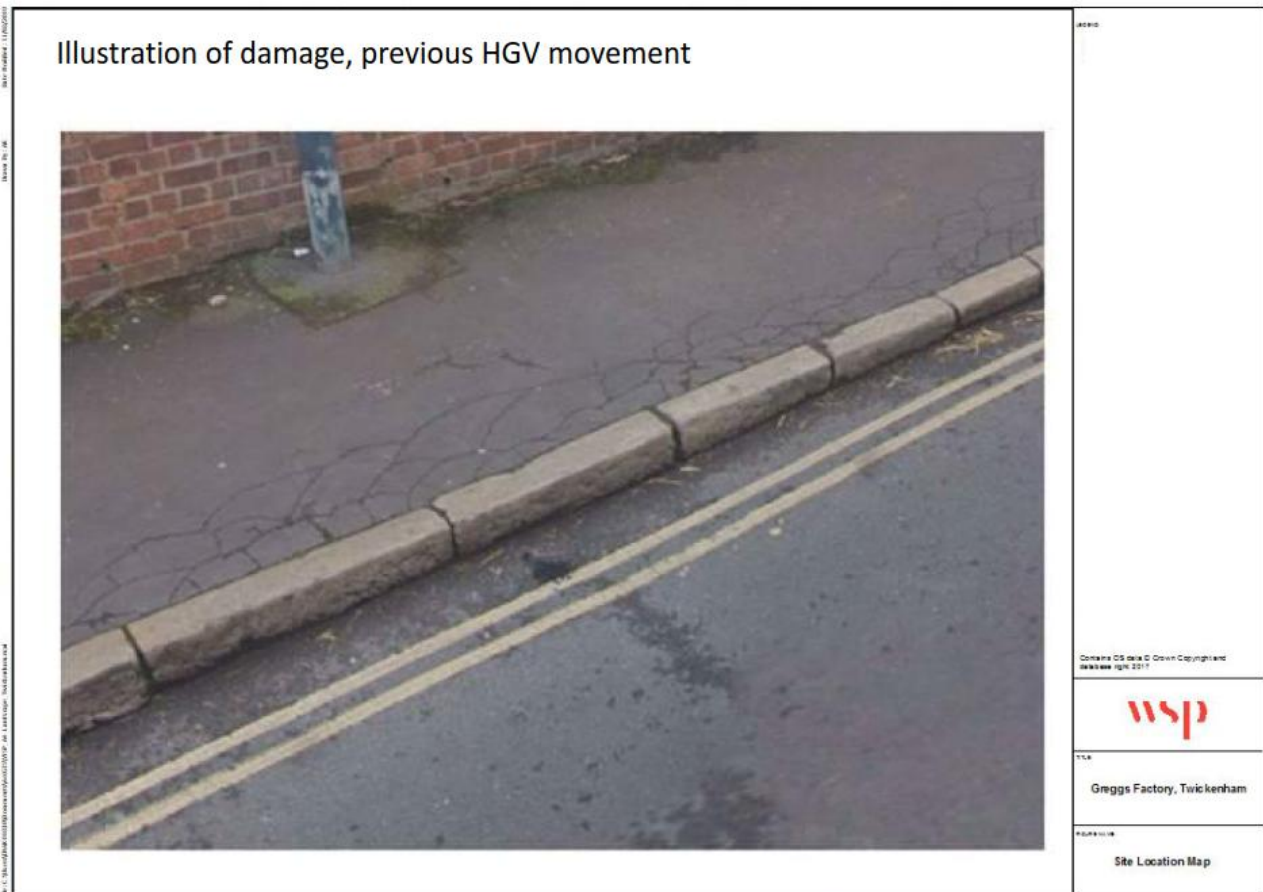
Figure 2 - Illustration of damage, HGV movement (Edwin Road and Marsh Farm Road)
