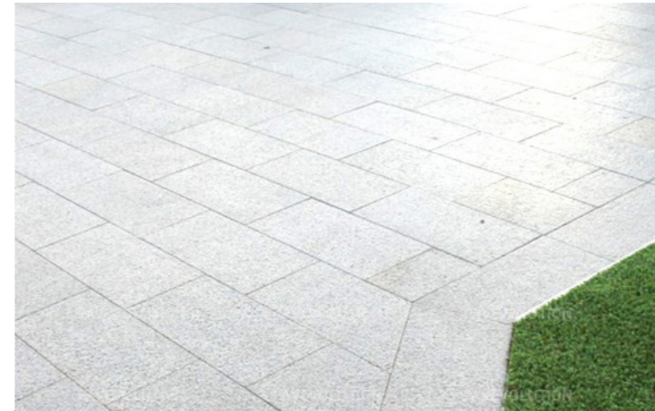
Granite paving with frame
