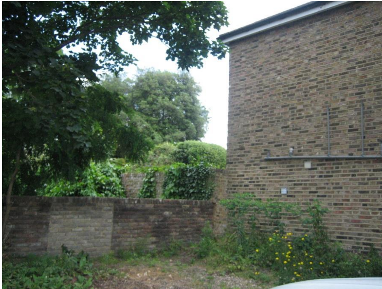
Figure 36: Wall dividing the land within the subject site which is part of no. 1 Spring Terrace from that which was formerly part of no. 2, and the north elevation of the extension to the house at no. 2 Mount Ararat Road to the right.
