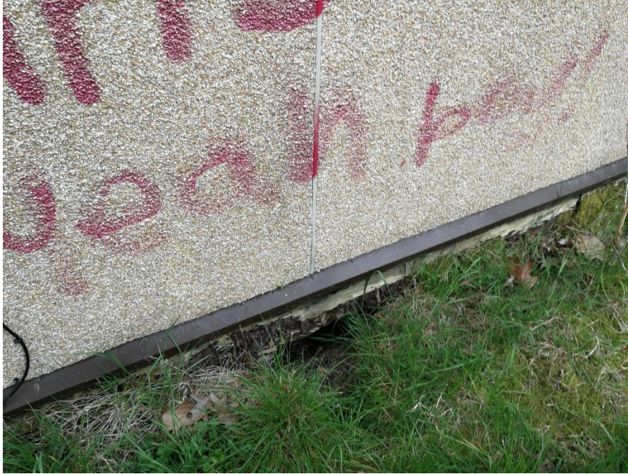
Photograph 18: entrance to the fox den under Building 3 at the Application Site.
