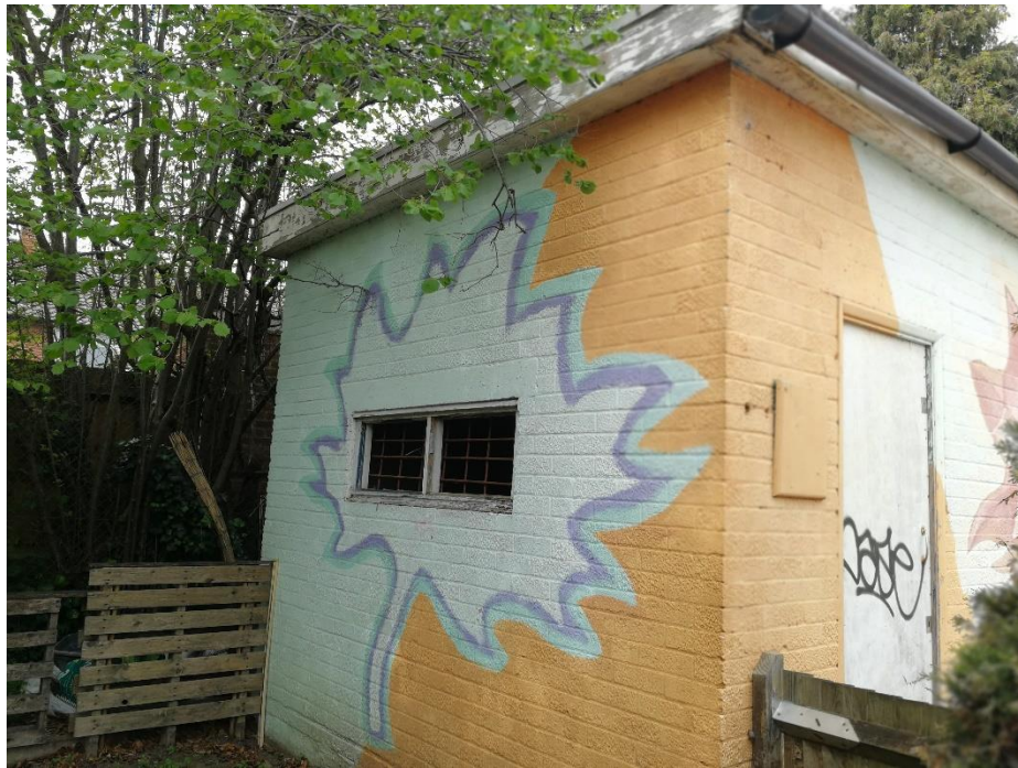
Photograph 4: View of Building 2 with the open window at the western border of the Application Site.
