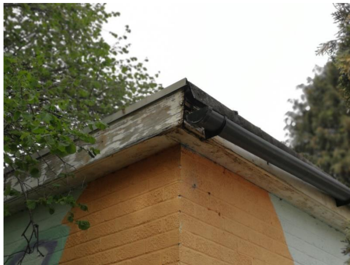
Photograph 16: Degraded soffit box on the corner of Building 2 on the Application Site.
