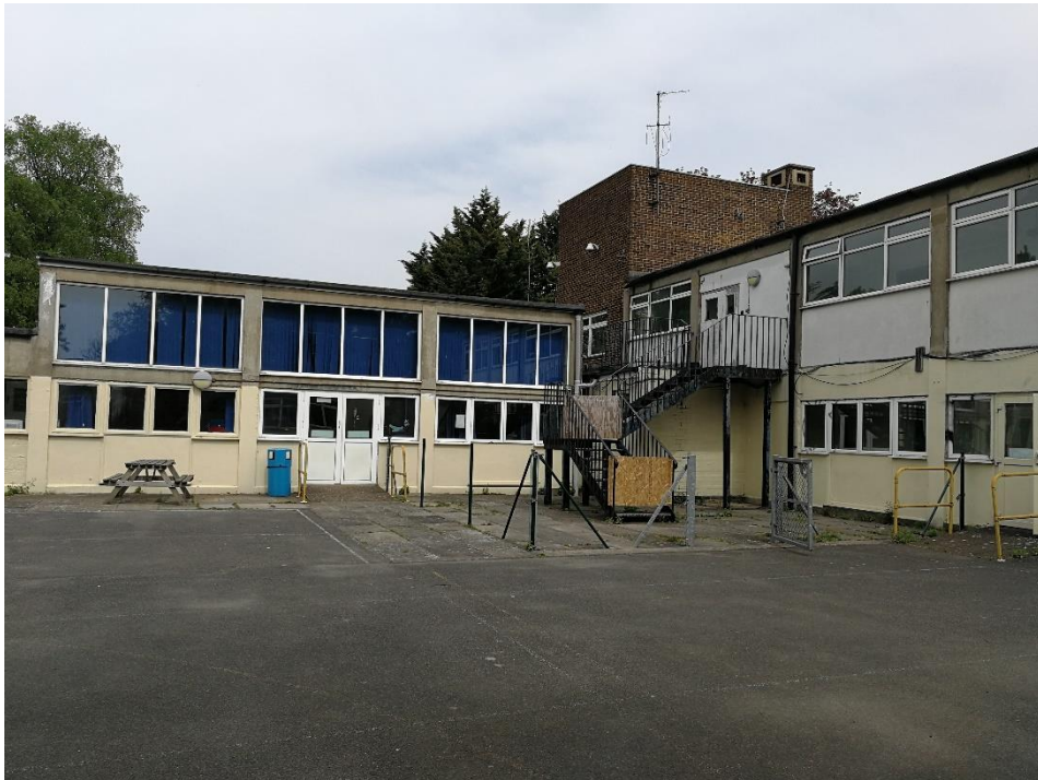
Photograph 3: View of hardstanding and western elevation of Building 1 at the northern end of the Application Site.
