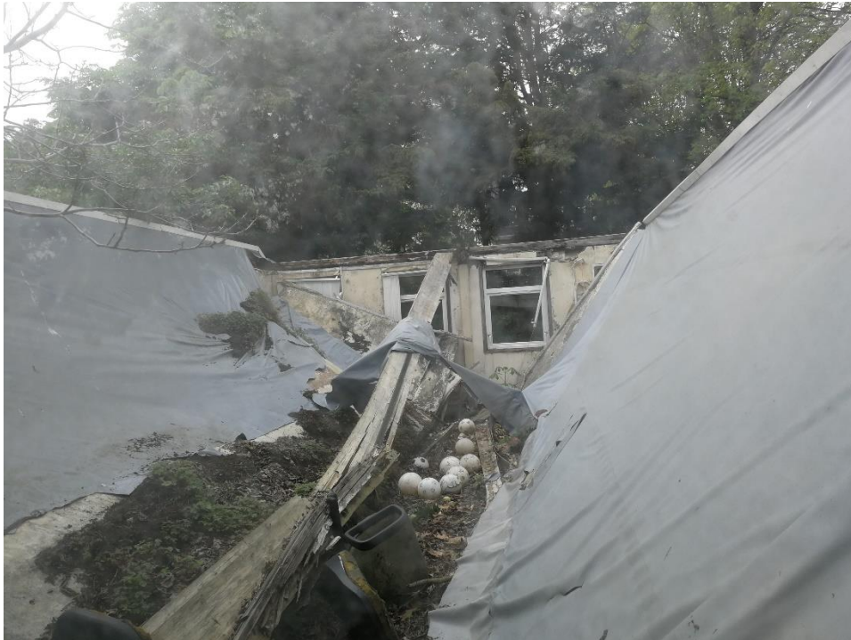
Photograph 5: View of the collapsed roof of Building 5 in the middle of the Application Site.
