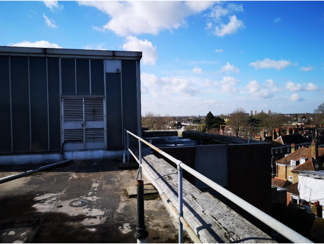
Figure 6 - View from roof / roof plant
