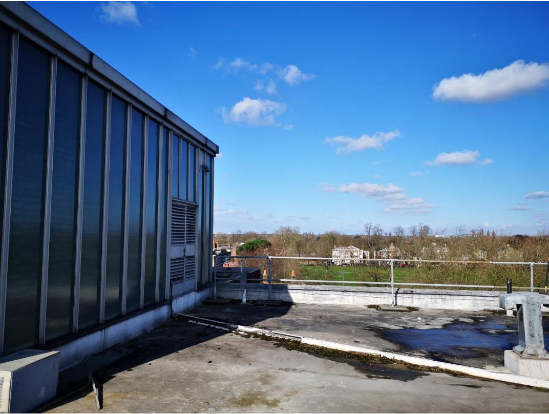
Figure 5 - View from roof / roof plant
