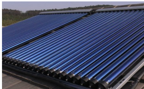
Figure 5 - Evacuated tube solar thermal panels
