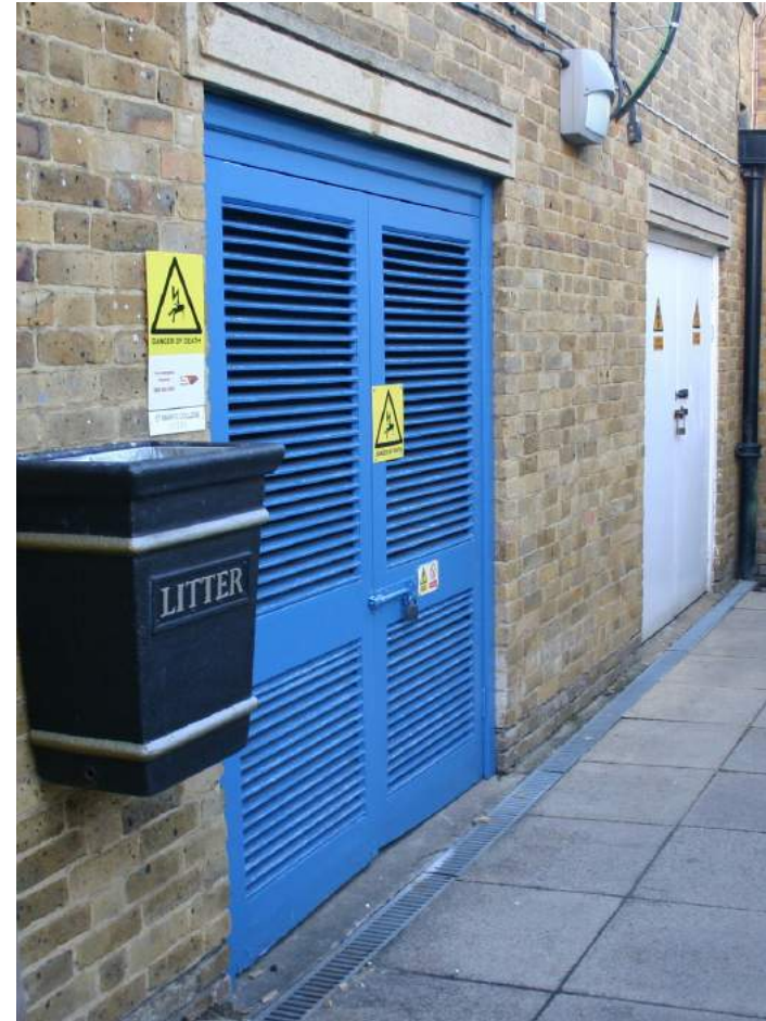
Substation in N Block
