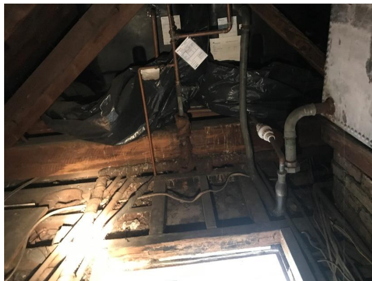
Plate 12 – Bird droppings within south-western loft space of building B10.
