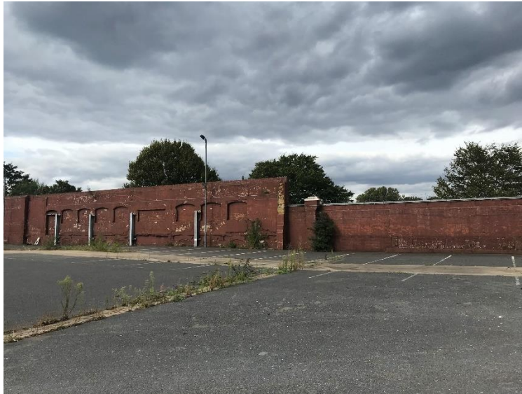
Plate 5 – Part of river wall along north-western boundary of the Site (Site side with River Thames beyond)
