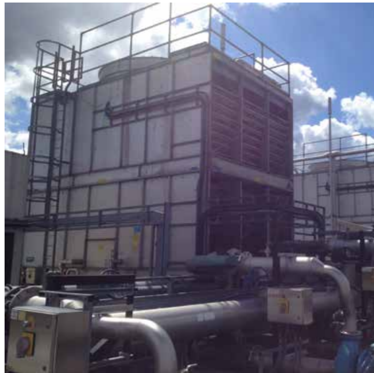
Air conditioners at The Power House Roof
