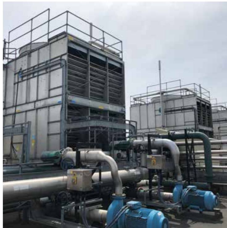
Air conditioners at roof of energy centre
