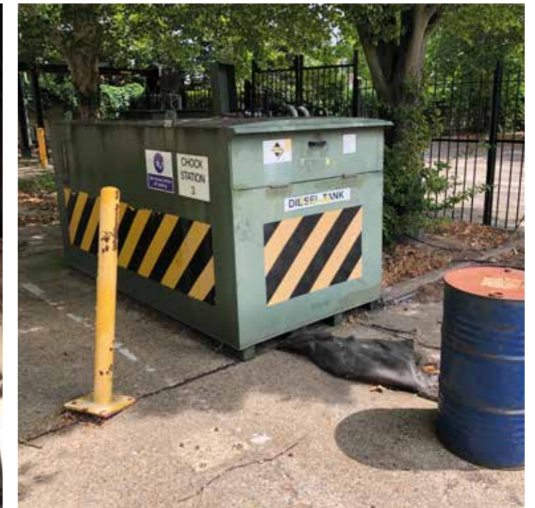
Diesel tank at north of eastern area
