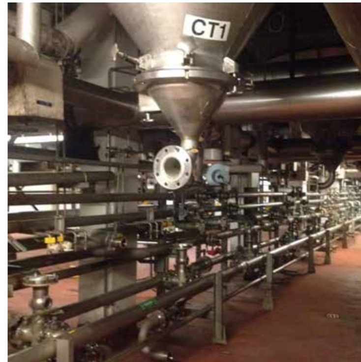
Brewery infrastructure in Brewhouse
