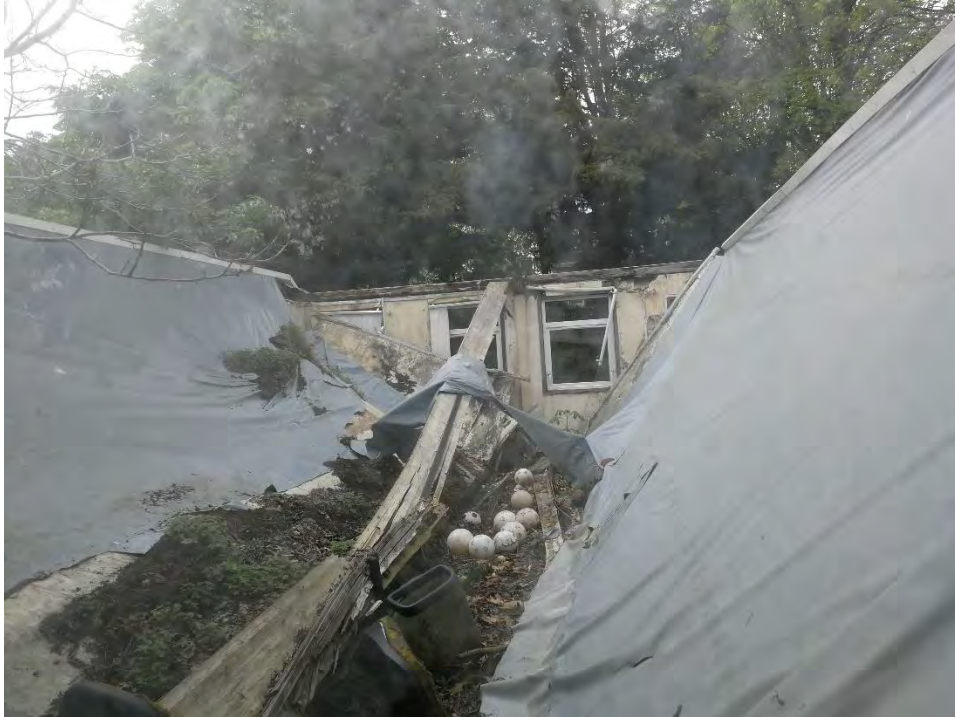
Photograph 5: View of the collapsed roof of Building 5 in the middle of the Application Site.
