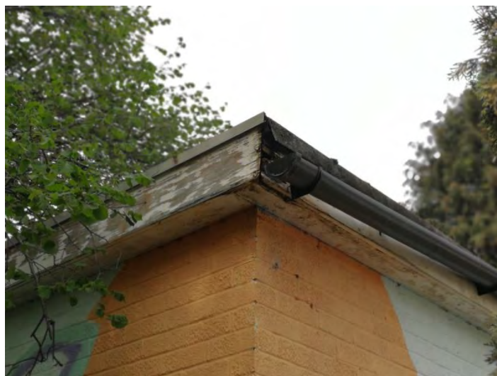
Photograph 16: Degraded soffit box on the corner of Building 2 on the Application Site.
