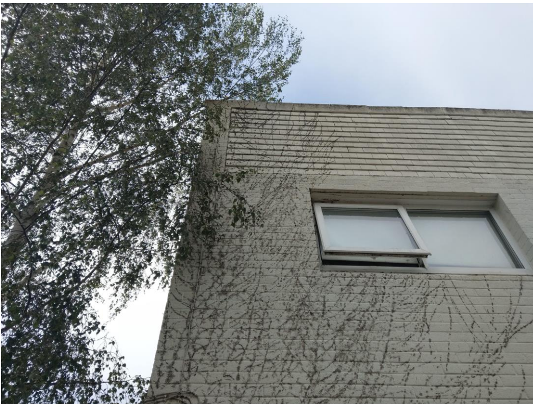
Photo A3.3: Rear (north east facing) of caretaker's cottage, gaps under roof tile
