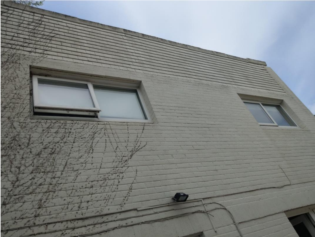
Photo A3.2: Rear (north east facing) of caretaker's cottage lifted hanging tiles in corner and gap under roof tile
