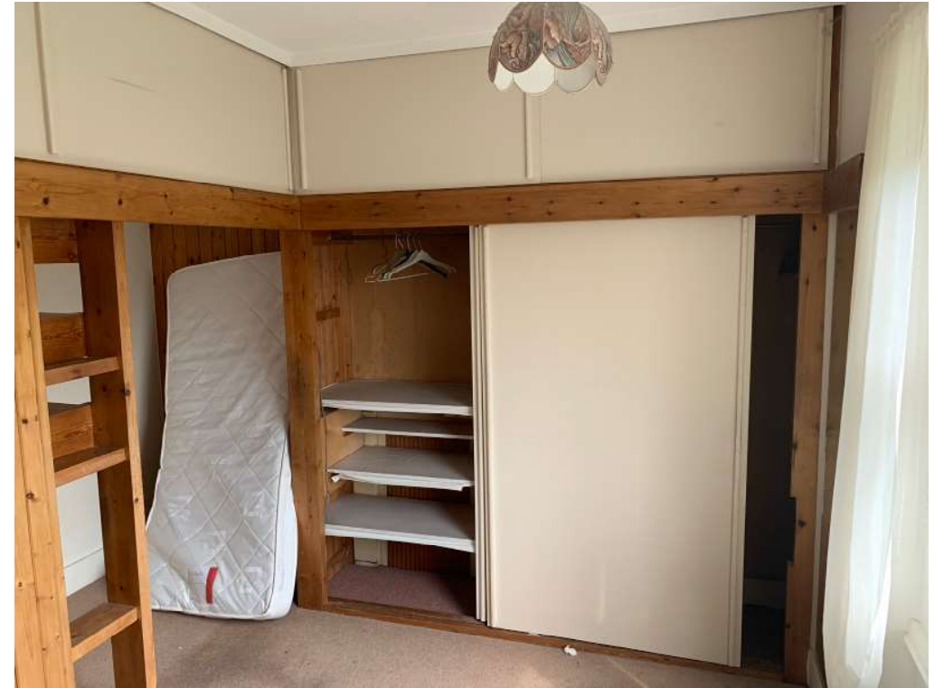
Figure 1: Each room had internal joinery built to divide further the space and conceal the original fireplace behind the fitted wardrobes
