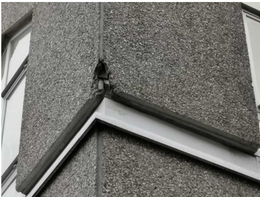
Plate 8: showing damaged rendering
