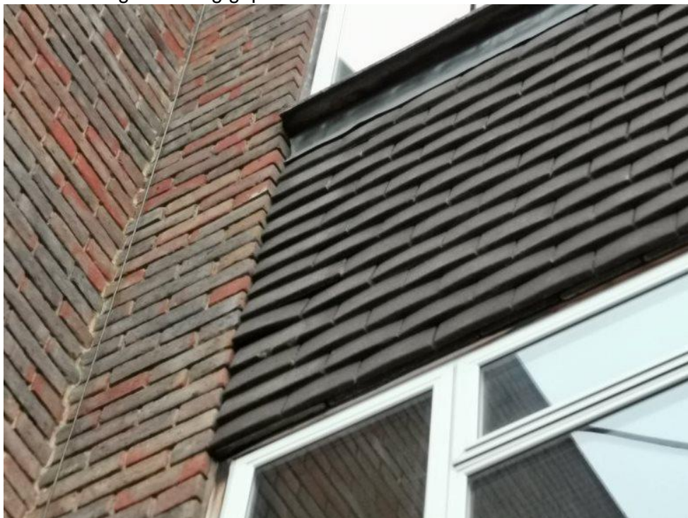
Plate 7: Image showing gaps under the tiles.
